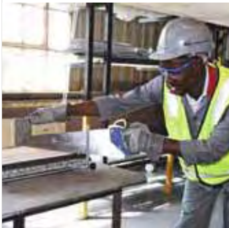
Gypsum - South Africa, Roodekop Factory and Training Center, gypsum plasterboard being sawed.
